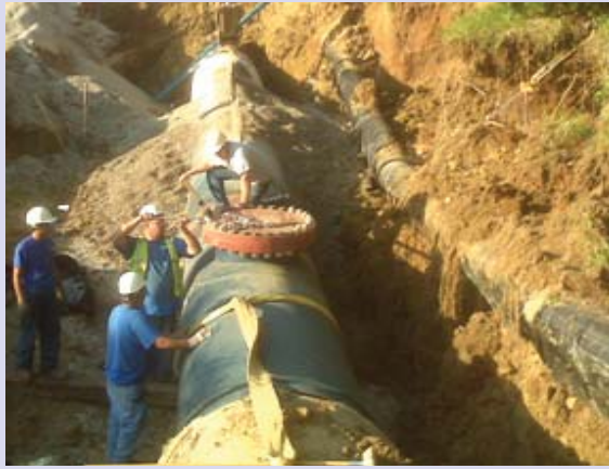
A WaterOne Construction & Maintenance crew working on repairing a 54" transmission main that ruptured the morning of July 1, 2011. Crews responded immediately to the large break and were able to restore water service to thousands of customers within the hour.
