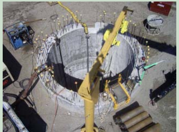
Photo showing aerial view of horizontal collector well.
