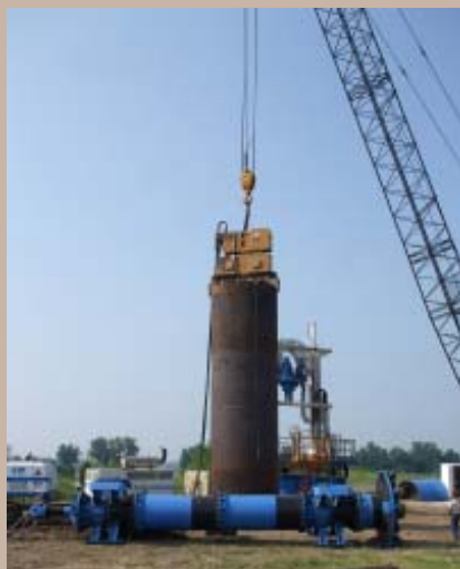
40-ft lengths of 9-ft diameter, 3/4" steel casing pipe being inserted into the shaft.
