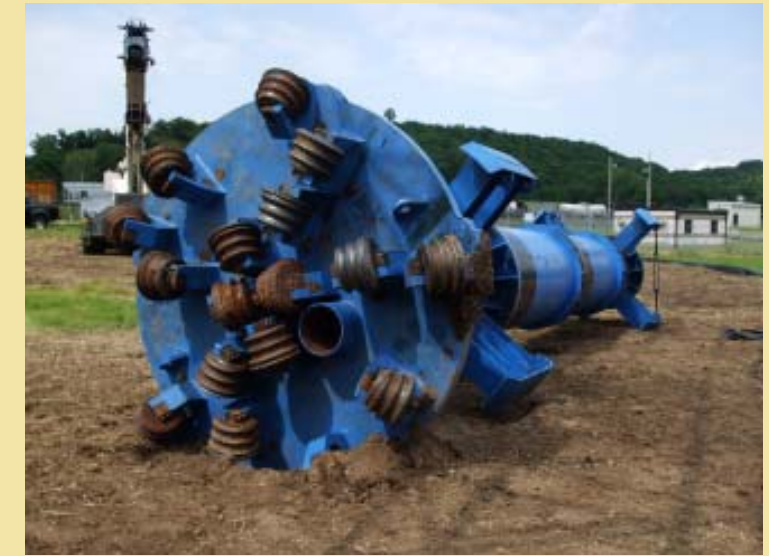
Drilling equipment used to drill shafts weighing over 10 tons. A 15-ton crane is required to maneuver the drill apparatus.
